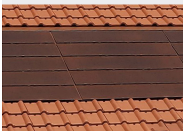
Integration von Photovoltaikmodulen
