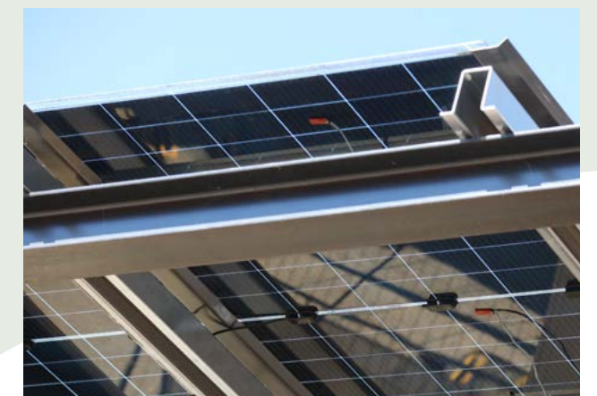
Monitoring der Photovoltaik-Leistung am STEP-Pavillon © Alejandro Paz (EPFL PL-MTI)
